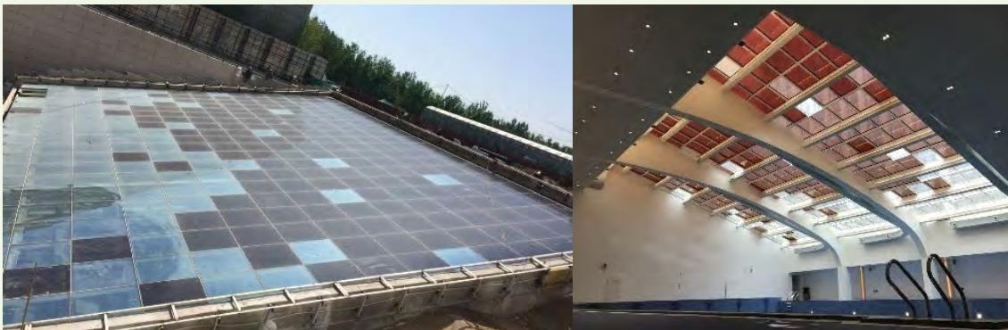
Solar Lighting Roof of Goldwind Swimming Pool 金風科技游泳池太陽能採光頂
