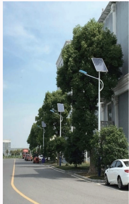
Outdoor solar street lights 室外太陽能路燈
