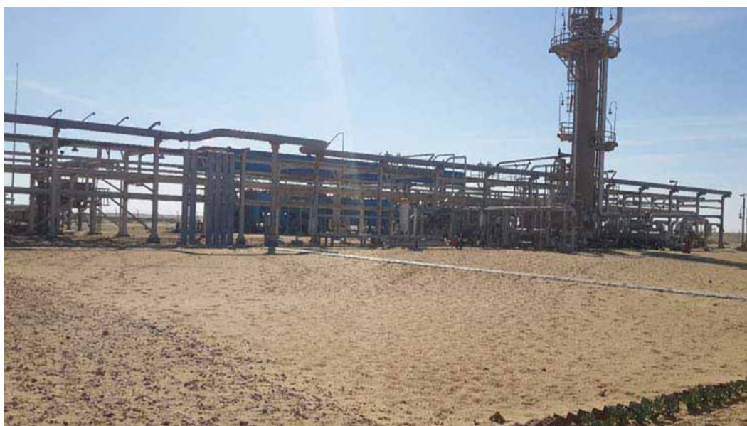
Figure AIII.14: General View of Gas Facility
