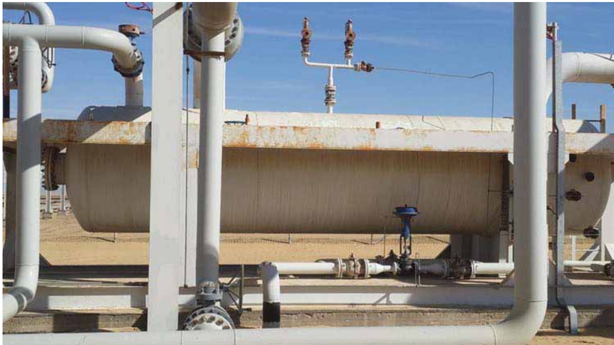
Figure AIII.15: FWKO Vessel and its Valves
