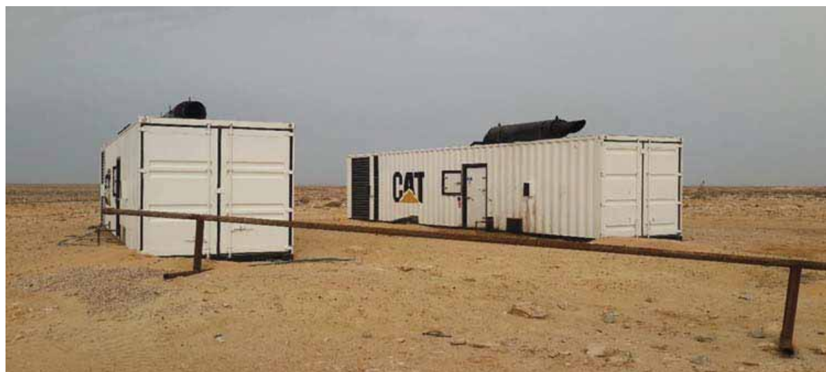
Figure AIII.6: CAT Generators
