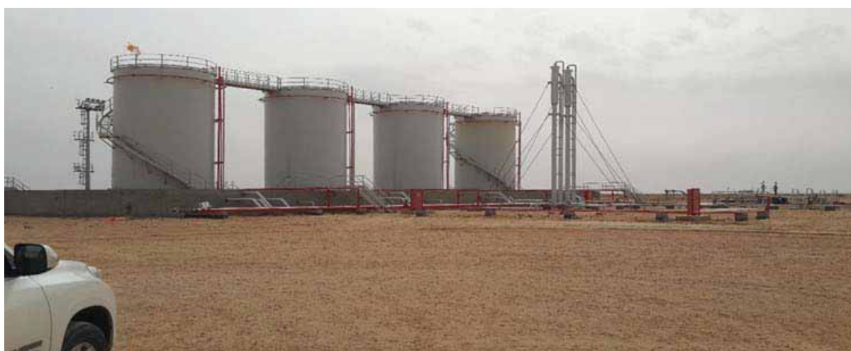
Figure AIII.1: Storage Tanks
