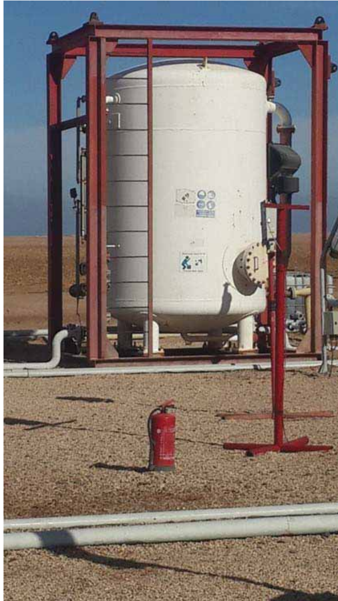
Figure AIII.20: Gas Scrubber
