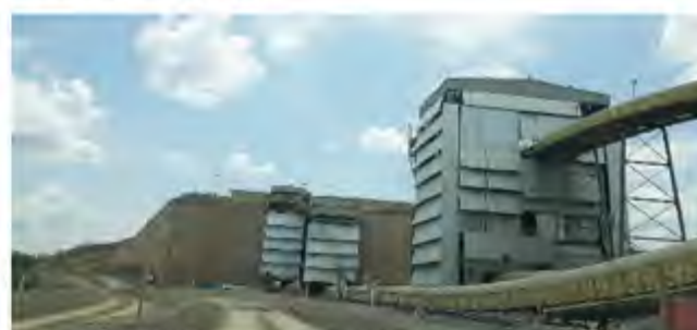
The enclosure of the crushing system of Boa Vista Mine was carried out in order to minimize the noise of the operation and minimize the emission of particulates to the atmosphere.
