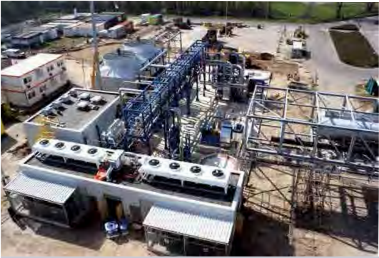
Dutch Enviro Energy commenced construction of Netherland's first large scale energy-from-waste CO 2 capture facility for greenhouse horticulture.
