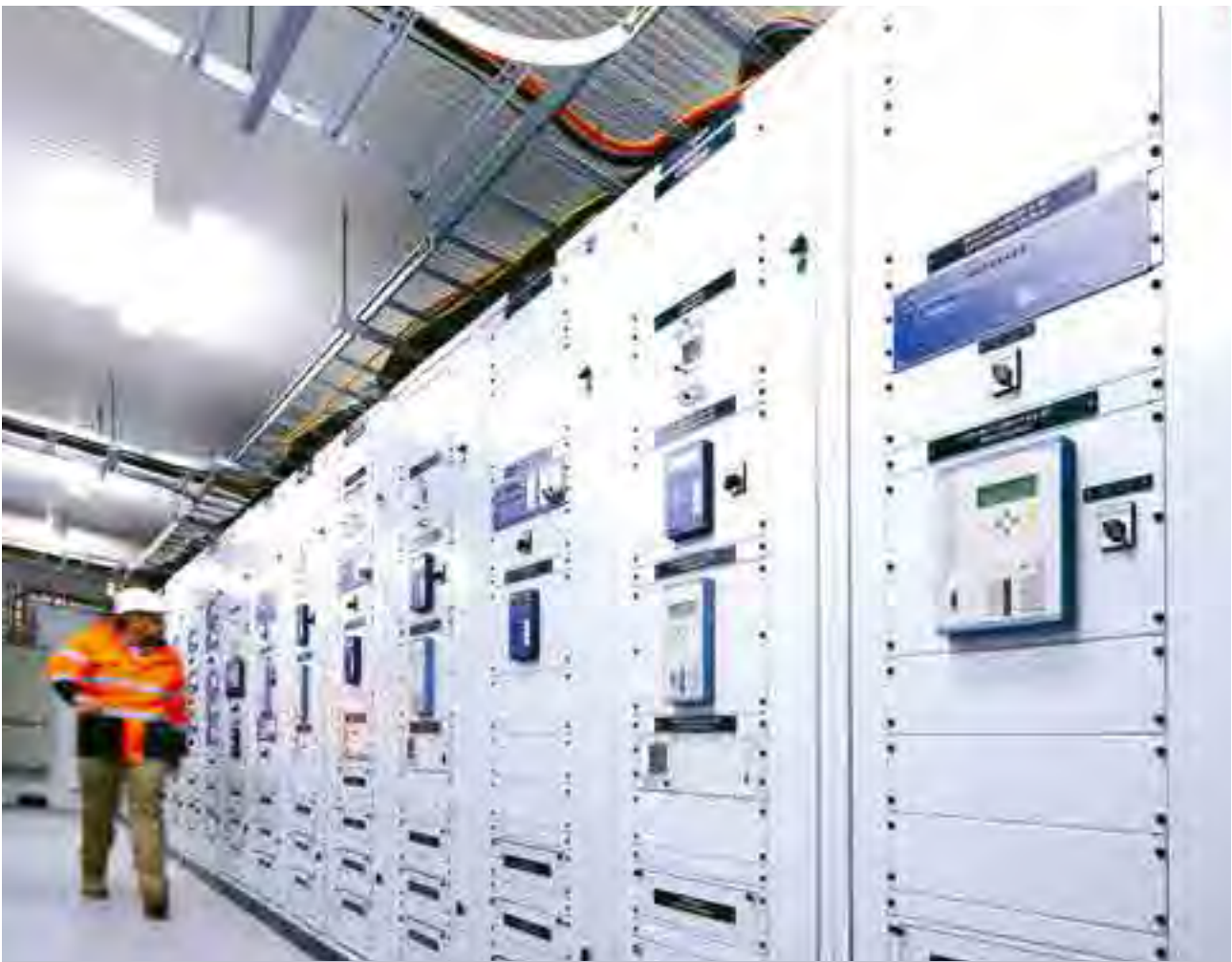
United Energy distributes electricity to approximately 688,000 customers across east and southeast Melbourne and the Mornington Peninsula.
