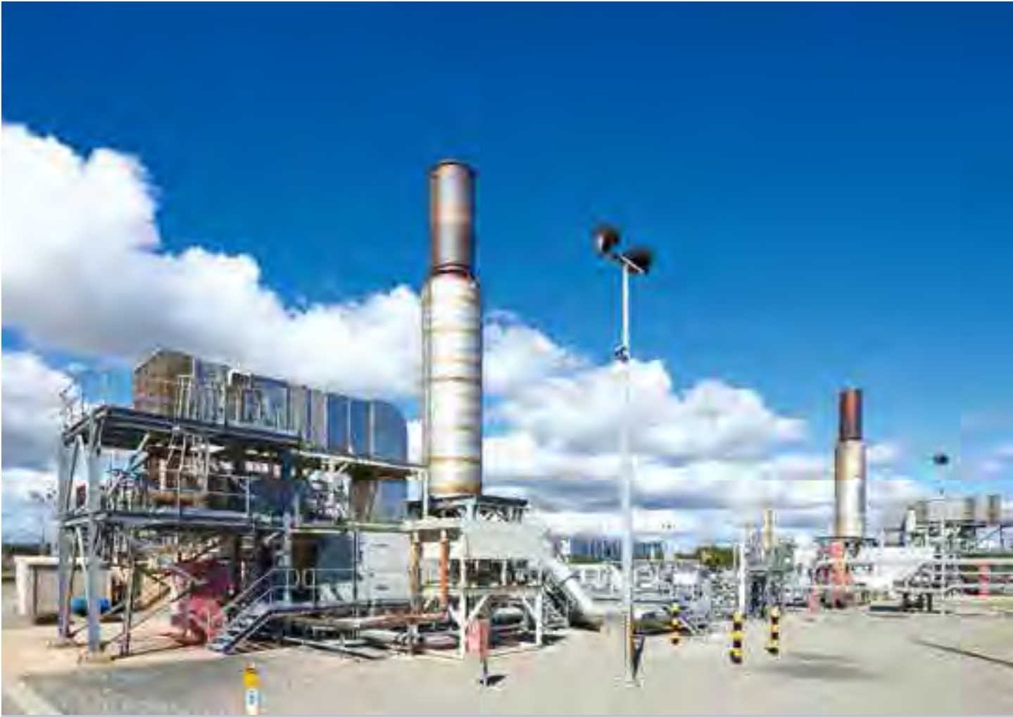
The Dampier Bunbury Pipeline stretches approximately 1,600 kilometres, transmitting the gas to mining, industrial, and commercial customers, as well as via other distribution networks to residential customers.
