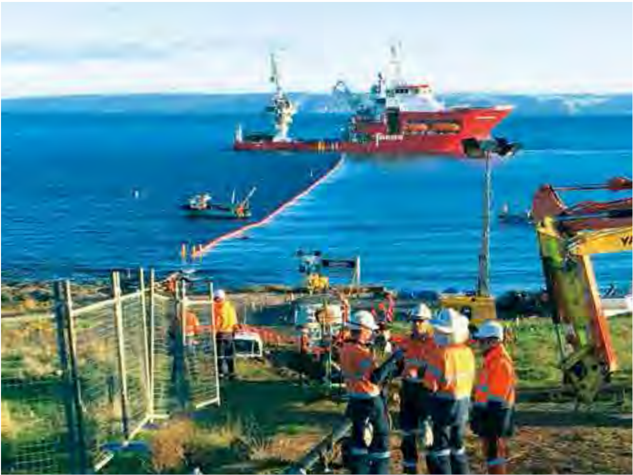
The replacement of the undersea cable connecting Kangaroo Island to the South Australia electricity distribution network was successfully installed.
