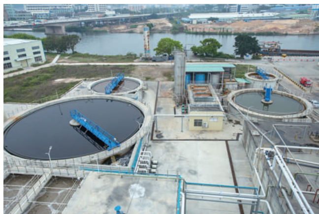
Zhongshan Rengo Hung Hing Papermaking Base has added a new environmentally friendly aerobic 5000 m 3 processing system
