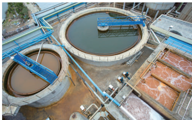
Zhongshan Yongfa Papermaking Base added 8000 m 3 semi-processing system for environmental protection new aerobic system
