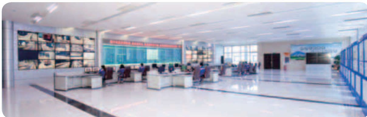
Control room of energy management center 能源管控中心主控室
