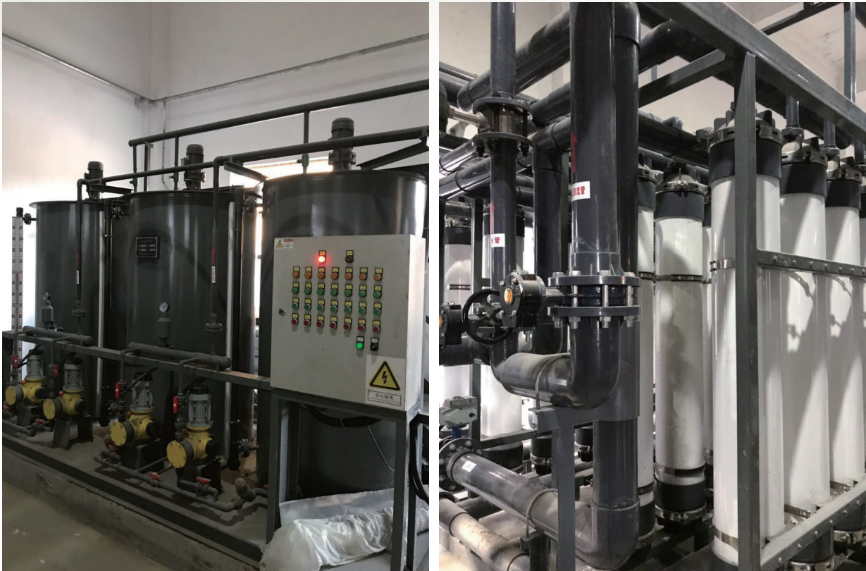
Mine Wastewater Treatment Facilities 礦場廢水處理設施
