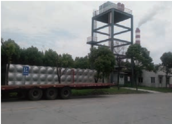
New fire system – water tanks and pump
