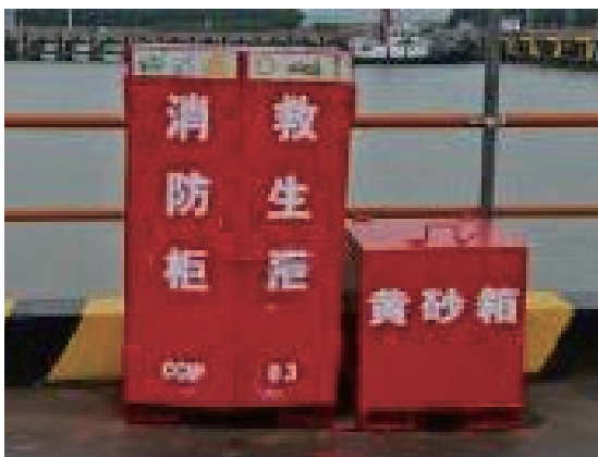
Fire and safety equipment cabinet after removal of rust and new paint work
