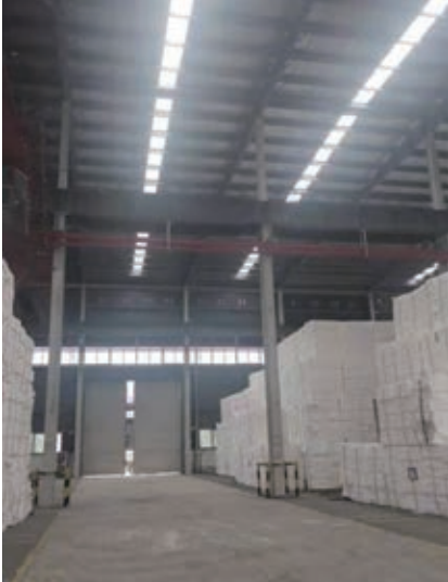
New fire system – fire hose
