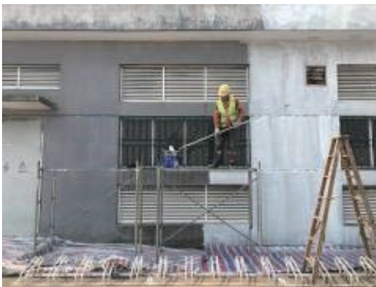
Electric power supply room – Before removal of rust and new paint work
