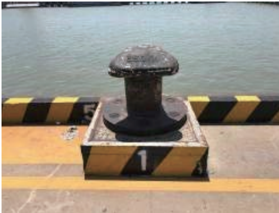
Bollard – Before removal of rust and new paint work
