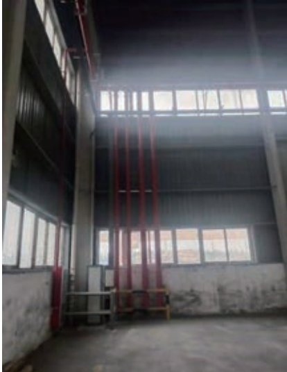
New fire system – fire hose
