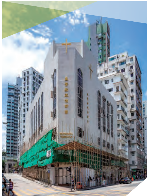
Renovation works for Pentecostal Mission Hong Kong and Kowloon Church at 71 Waterloo Road 窩打老道71號港九五旬節會教堂之裝修工程
