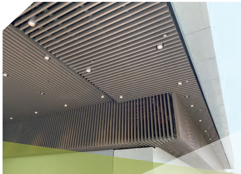
Design, supply and installation of external ceiling system for West Kowloon Government Offices at Yau Ma Tei 油麻地西九龍政府合署－設計、供應及安裝外部天花系統
