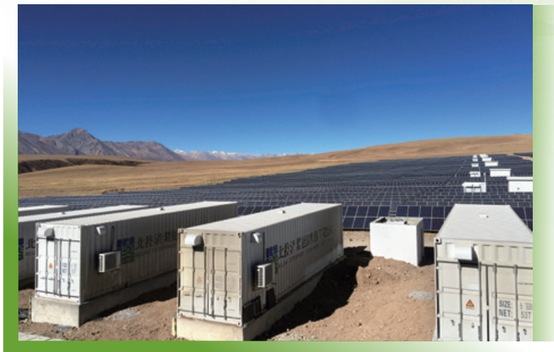
Yangyi Photovoltaic Energy Storage Project, the Tibet Autonomous Region 西藏自治區羊易光伏儲能項目
