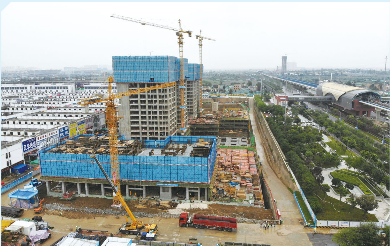
The multi-purpose office and apartment complex –1668 Square under construction next to subway station 在建的多功能商辦及公寓綜合體 –1668廣場鄰近地鐵站口
