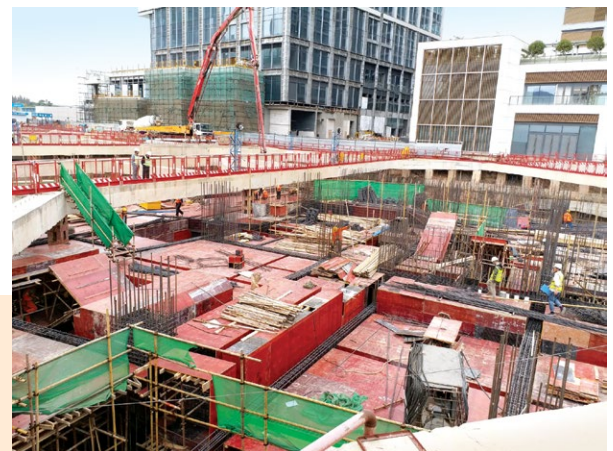
The future location of BEA's GBA Headquarters in Qianhai, Shenzhen, which is currently under construction.
