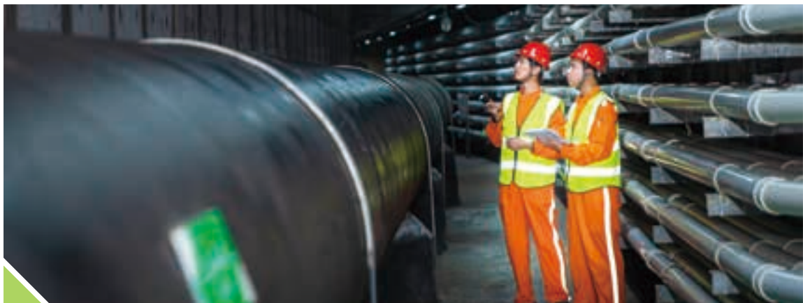
The underground comprehensive pipeline corridor located in Hengqin is 33.4 kilometers long. This photo shows staff carry out daily inspection inside it.
