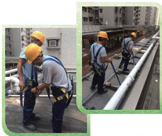
Demonstrated the proper application of steel wire anti-drop protection device 演示防墮鋼索保護裝置的正確使用方法
