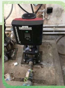
The variable frequency water pump installed in the pump room 我們在泵房中安裝的變頻水泵
