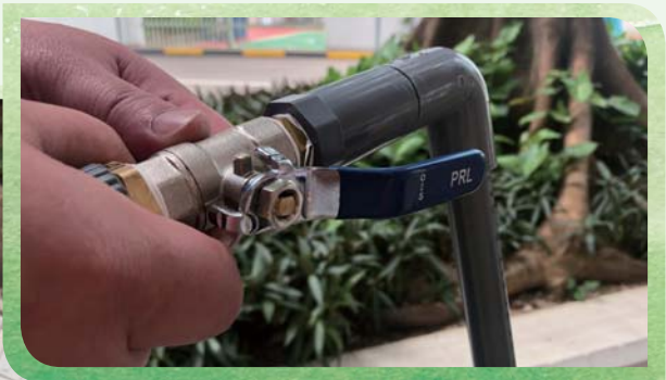
Connecting the water pipe to the flush pipe 把水管連接到沖洗管
