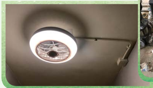
The ceiling-mounted luminaires equipped with a fan that provides luminance together with ventilation 配有風扇以作照明和通風的吊頂照明設備
