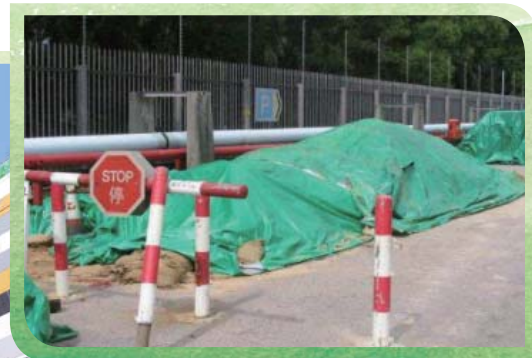
Our site workers used impervious sheeting to cover stockpiles of dusty materials 我們的地盤員工以防水布覆蓋堆放著的多塵物料
