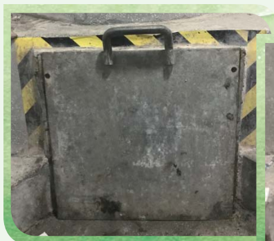
The refuse chutes shutters shall always remain closed 垃圾槽的擋板保持常關
