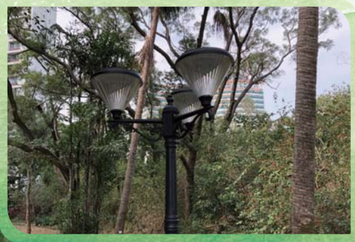
The solar panel installed onto the pole lights 安裝在燈柱的太陽能電池板
