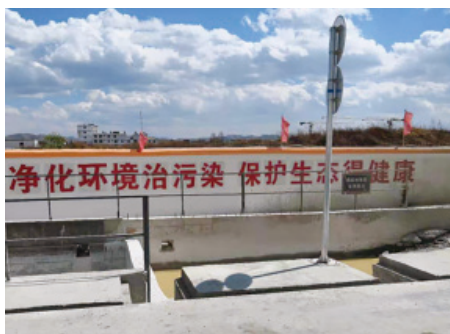
Sewage tertiary sedimentation tank 污水三級沉澱池
