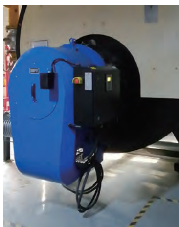
Low nitrogen boiler
