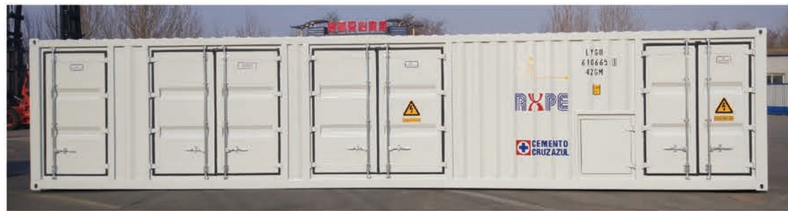
A container-turned substation
