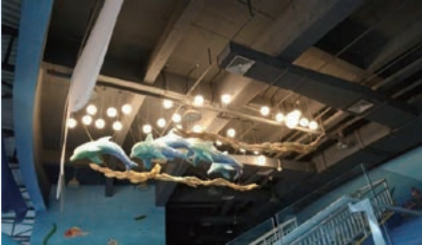
Revamped LED landscape lighting 改造LED景觀燈
