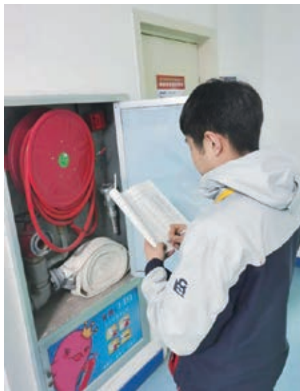
Carbon-dioxide and dry-powder fire extinguishers were replaced in Qingdao Haichang Polar Ocean Park to eliminate potential fire hazards
