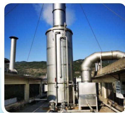
福州統一油煙淨化系統餘熱回收 Heat recovery from the oil fume purification system in Fuzhou President
