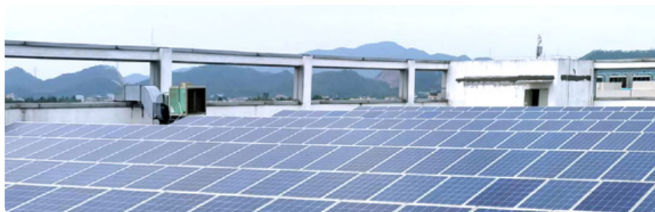
Solar photovoltaic power generation project
