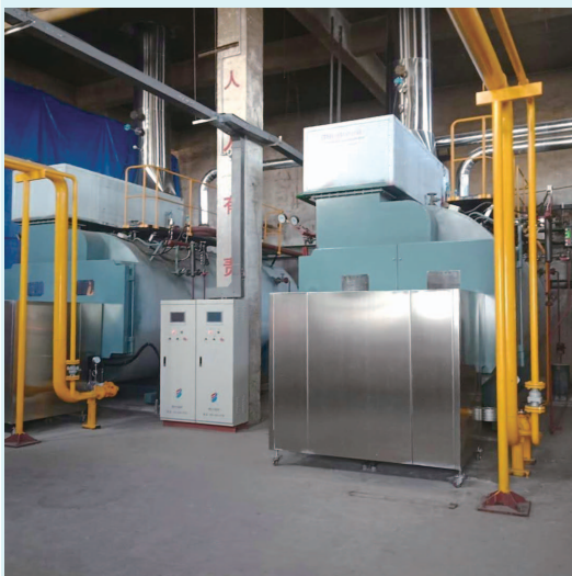
燃氣鍋爐 Gas-fired boilers
