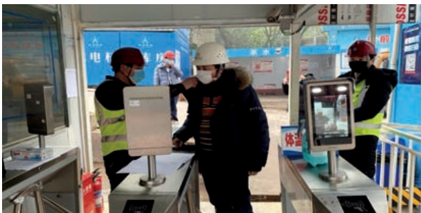
Measuring and recording employees' temperature twice a day, and setting up disinfection corridors at entrances and exits of buildings and construction sites. 每天兩次為員工測量及登記體溫，在大廈及地盤出入口設置消毒通道。
