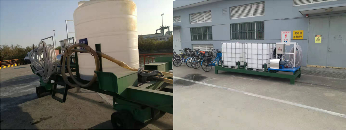
Barges sewage collection and distribution
