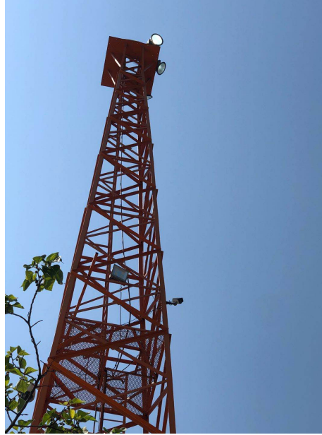
16 sets of 600W LED light posts at stack yards
