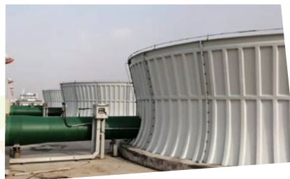
循環水站 Water recycling station
