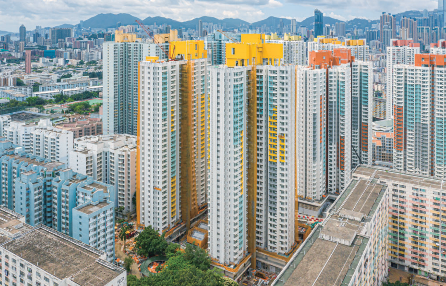
Construction of Public Rental Housing Redevelopment at Pak Tin Estate Phases 7, 8 and 11 白田邨第七、第八及第十一期公共租住房屋重建項目建築工程
