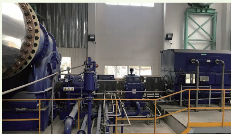
Sulfur Dioxide Fans after Transformation
