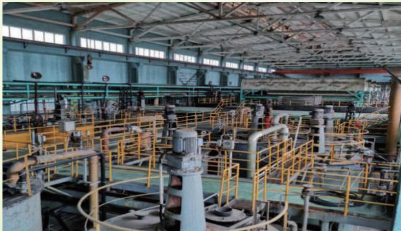
Arsenic Trioxide Production Facilities
