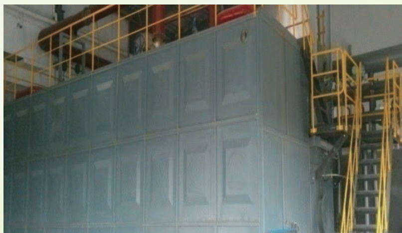
Gas Furnaces after Transformation
