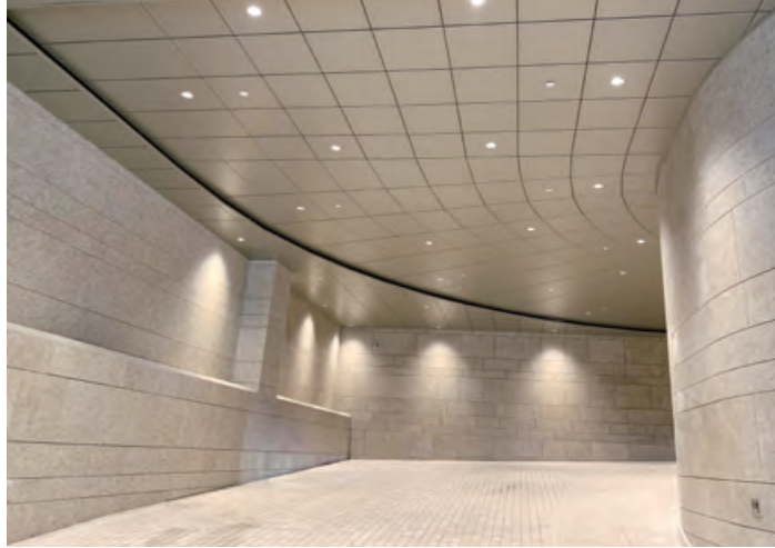
Supply and installation of external ceiling system for residential redevelopment at No.23 Robinson Road at Carpark 羅便臣道23號之住宅重建項目（停車場）－供應及安裝外部天花系統
