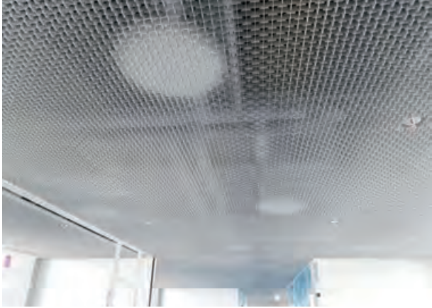
Supply and installation of metal ceiling and FRP system for Museum Plus (M+) at West Kowloon Cultural District 西九文化區 Museum Plus (M+) – 供應及安裝金屬天花及防火天花系統
