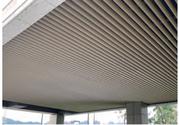
Supply and installation of suspended ceiling system for Lohas Park Package 7A & B 日出康城第7A及7B期 – 供應及安裝假天花系統
