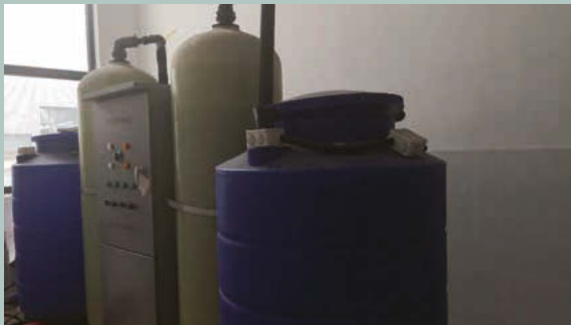
Xuzhou Baolan wastewater tertiary purification tank
