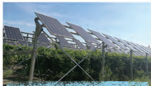
Photovoltaic + Viticulture 光伏+葡萄種植
