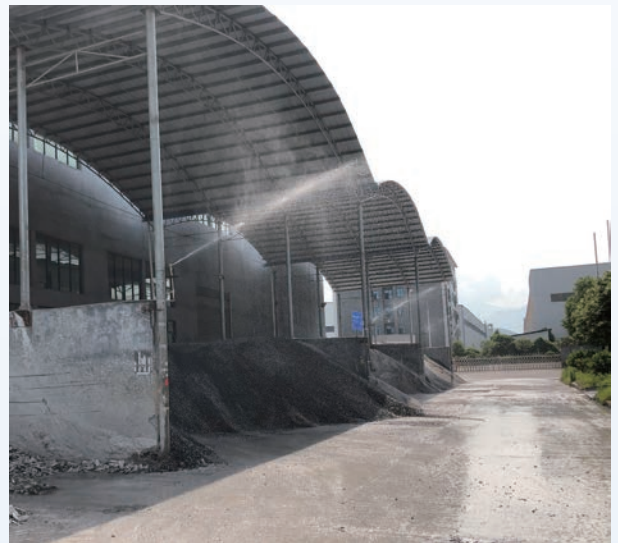
Picture 1: Spray dust reduction facilities in Lugu No. 2 Factory in Changsha
