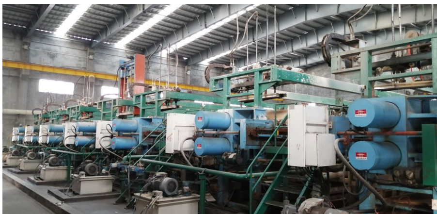
Sludge recycling equipment 污泥回收設備
