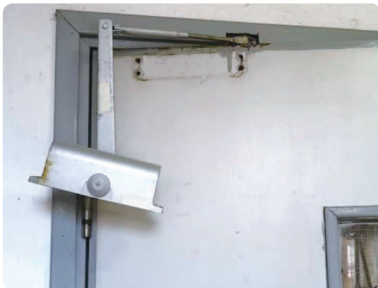
Before Repair 維修前
