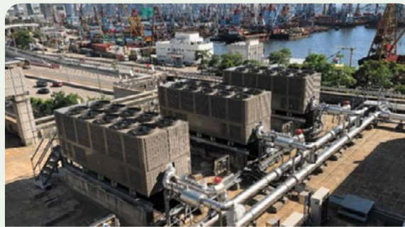
Chiller Plant at Olympic Station
