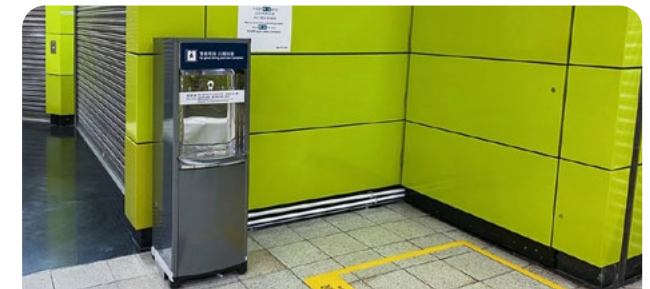
Water dispensers installed at stations to encourage the use of reusable water bottles
