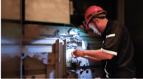
電梯服務 Elevator Services
