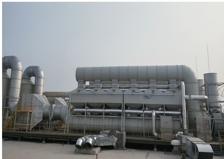
Waste Gas Treatment System of Bazhou Factory 霸州工廠的廢氣處理系統
