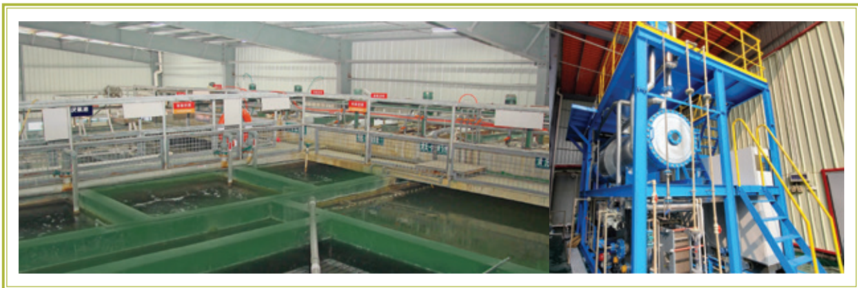
Wastewater treatment systems and grey water recycling system 廢水處理系統及中水回用系統
