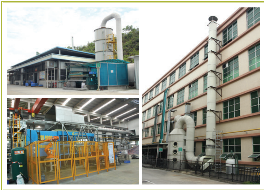
Air purification system and waste gas treatment system 空氣淨化系統和廢氣處理系統
