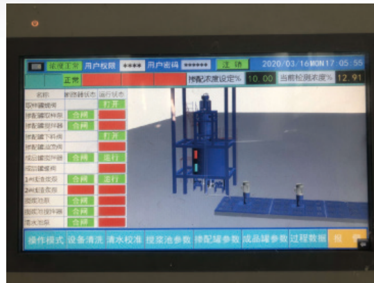
Real-time monitoring screen of seriflux recycling system 漿水回收系統實時監控畫面
