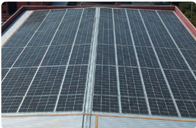
寧波廠區的太陽能發電板 PV panels in the Ningbo factory area
