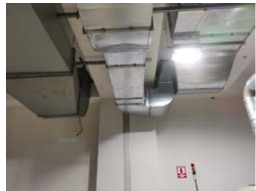
Ventilation devices in the basements of the CMTR-1 plant
