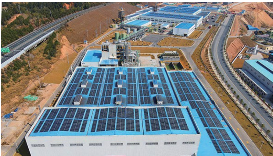
Zijin New Energy's first 3.4MW distributed photovoltaic power generation project has been put into use
