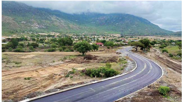
Nkwe's Garatau Platinum Group Metals Mine repairs and builds roads for local communities
