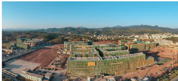
View of the actual construction site of Zijin Secondary School's new campus
