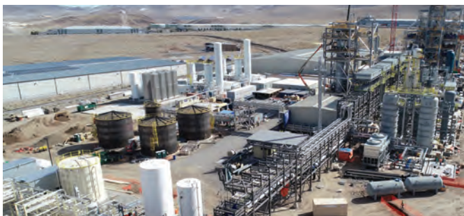
Fulcrum bioenergy plant construction, November 2019. The plant is progressing well and is expected to be completed in 2021.
