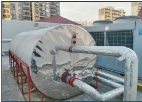
Energy-saving transformation results of air source heat pump hot water system
