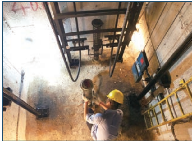
Elevator maintenance, repair and inspection
