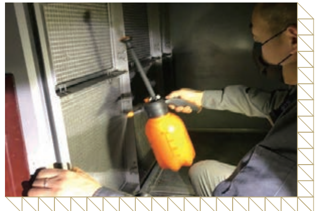
Sanitising filtration system
