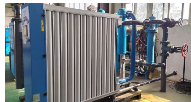
空壓系統模組式乾燥機節能技術應用 The application of energy-conserving technologies in air compressed modular dryer
