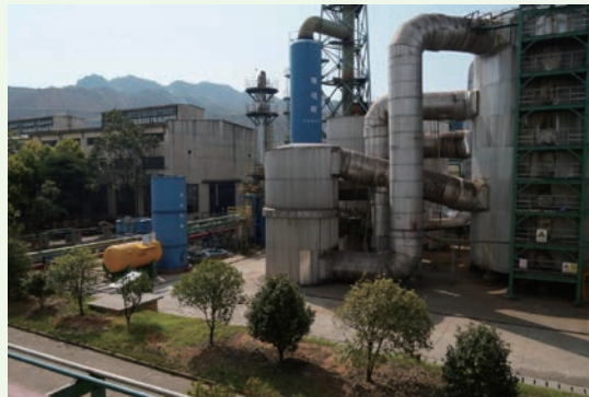
離子液法脫硫吸收塔 Ion liquid desulfurization absorption tower
