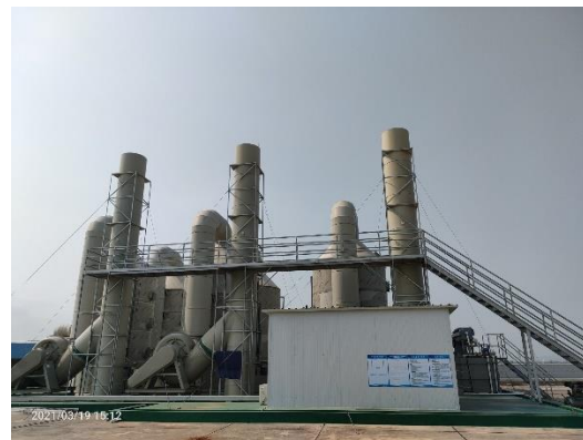
Acidic Mist Exhaust Treatment Facilities
