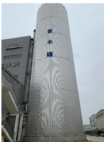
Water Storage Tank – cold energy storage / air-conditioning equipment
