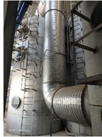
Spraying Tower for handling of paint exhaust
