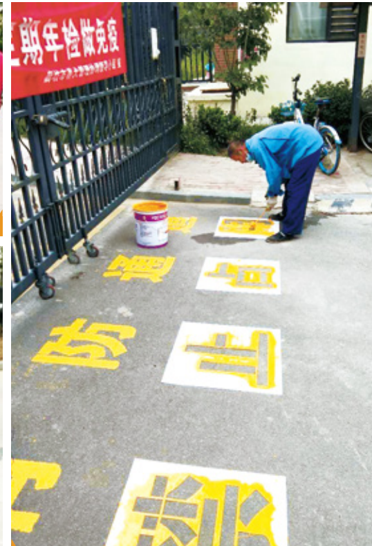
Marking Emergency Exits
