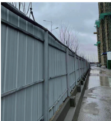
Sprinkling along the fence 圍牆端部佈置噴淋
