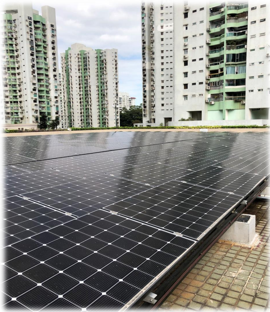
Solar Energy Equipment at Ocean Gardens
